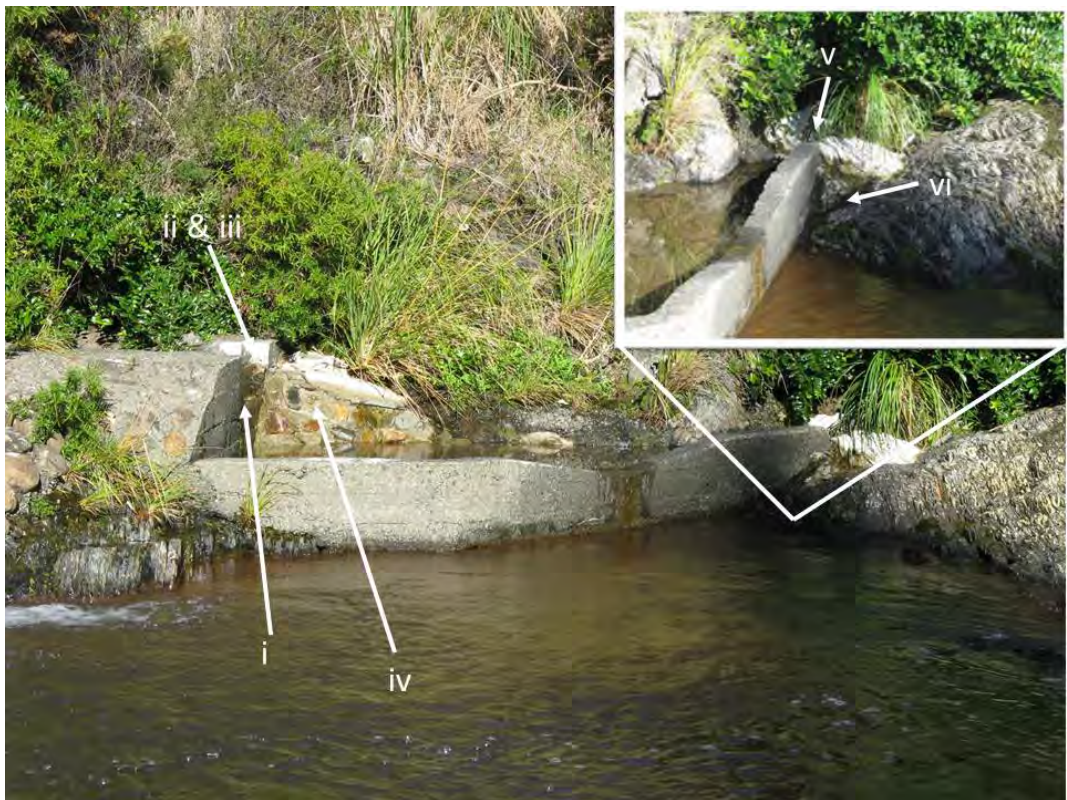
Figure 3. Step-pool fish pass on true left of the Maitai South Branch weir, following remediation work. Numbered arrows indicate remediation undertaken, with numbers referring to the points outlined under heading 3 of the recommended remediation actions in section 2.1.1, above. Note: river flow in this image is substantially lower than in Figure 2.
