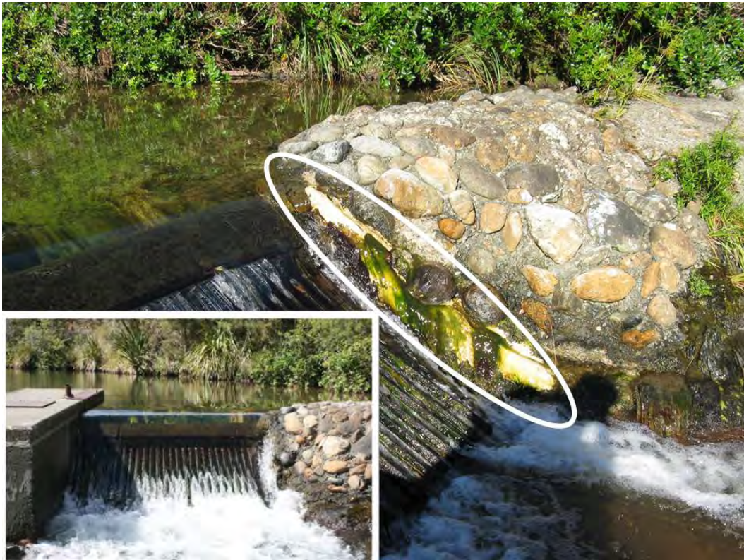
Figure 4. The water intake screen in the Maitai South Branch weir, showing the smooth wetted margin constructed with epoxy cement as part of the remediation works (highlighted within the white oval). Insert shows the screen prior to remediation.
