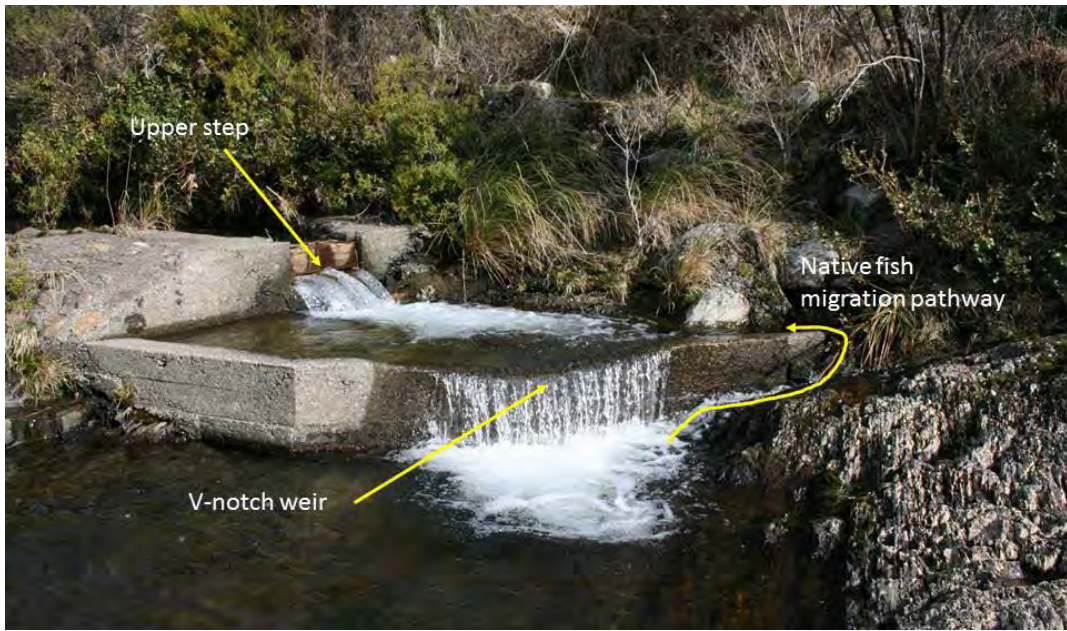
Figure 2. Step-pool fish pass on true left of the Maitai South Branch weir, prior to remediation work.
